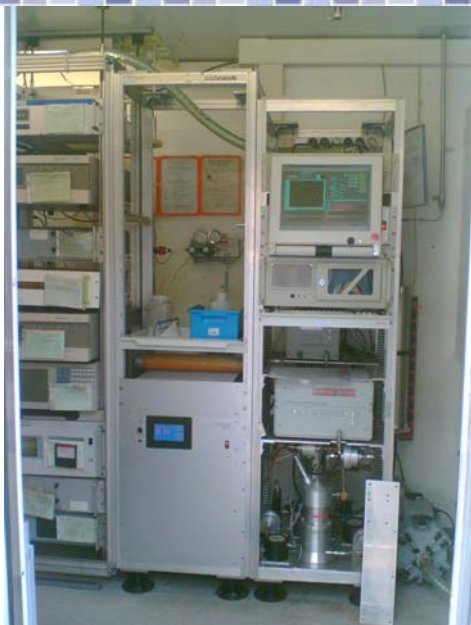
Fig. 4 26-06 – 09-07-2006 First test runs in the measuring station Dresden (Photo: UBG).
