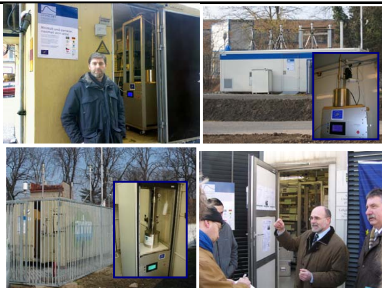
Fig. 8 Info plates and running instruments at all 4 stations Feb-2007: Stockholm (up, left), Augsburg (up, right), Prague (down, left), and Dresden (down, right) (Photos: ITM, GSF, CHMU, lft, LfUG).
